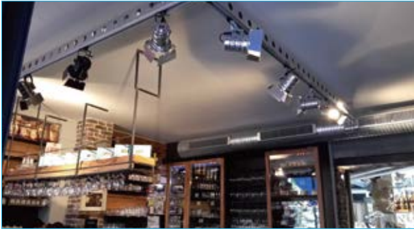
Trattoria Restaurant U-Match; Duct France
